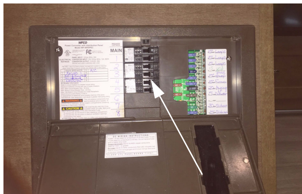
120-Volt Circuit Breakers -Typical View
