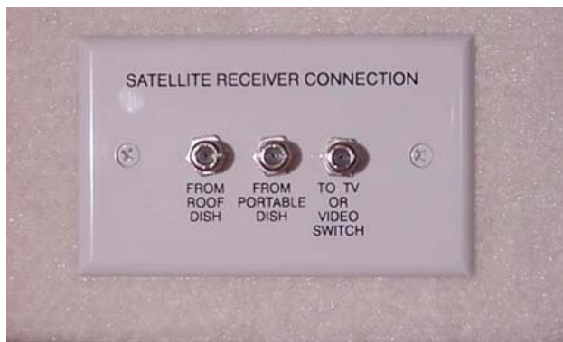
Interior Connection for Satellite Dishes (Located in cabinet near TV) Typical View
