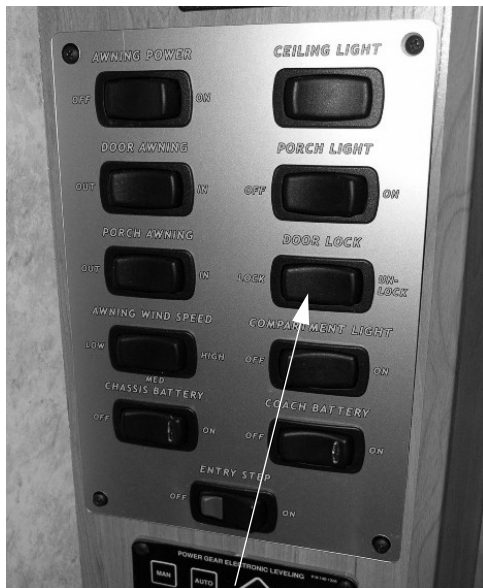
Power Door Lock Switch (Located near entrance door) -Typical View
