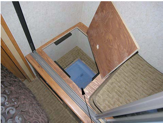
AC/Furnace Filter under wardrobe floor panel
