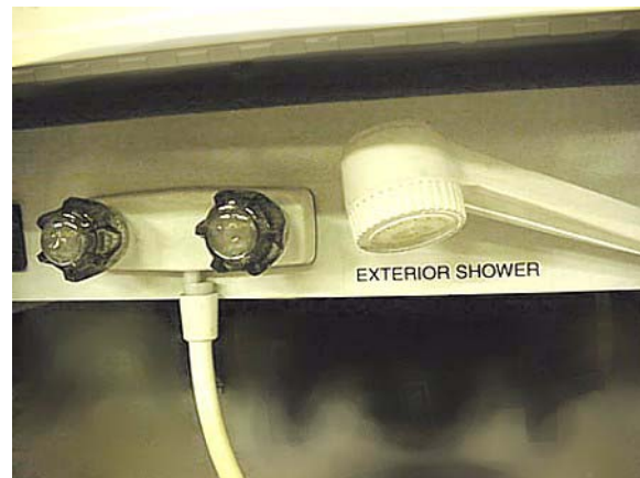
Exterior Shower/Wash Station -Typical View
