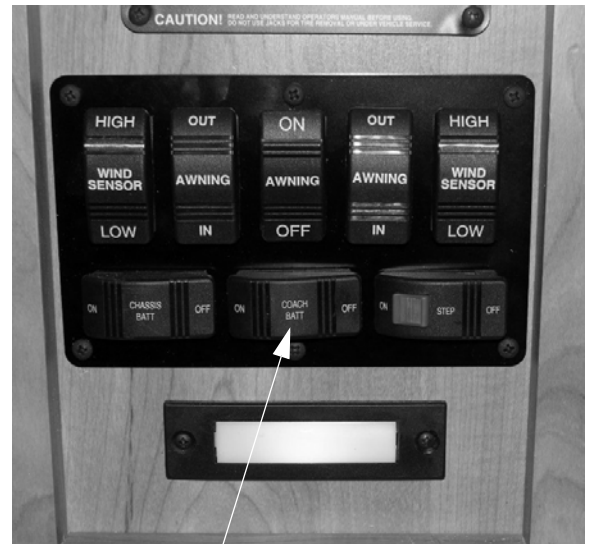
Auxiliary Battery Switch (Located near entrance door)
