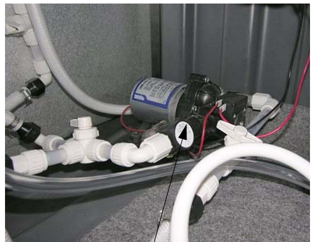
Water Pump (Typical)
