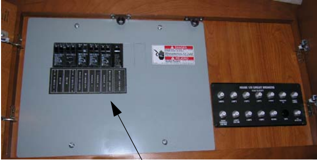
House 120-Volt AC Circuit Breaker Panel
