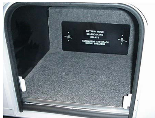
Chassis and House 12V Breakers in exterior storage compartment (remove cover to access)
