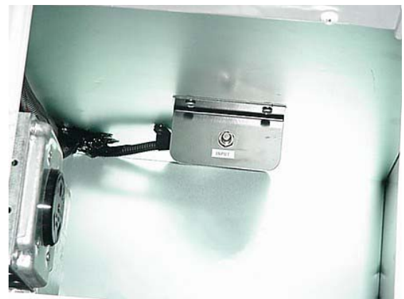
Cable TV Hook-Up in Utility Compartment
