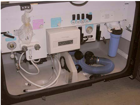
Water Service Center - typical view
