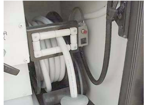
Water Hose Reel
