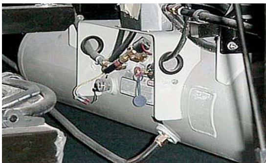
Propane Gas Tank behind slideout room
