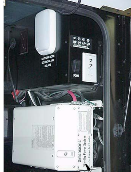
Inverter Charger Unit Location in utility compartment
