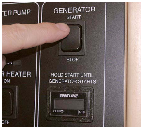
Generator Switch and Hourmeter on monitor panel
