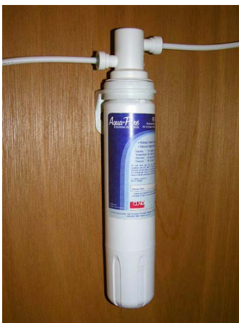
Water Filter Assembly (Located below galley sink)
