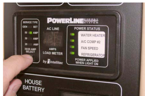
PowerLine EMS Display on Monitor Panel - typical
