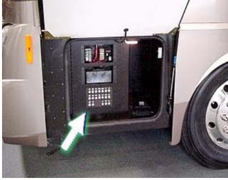
12V Electrical Compartment
