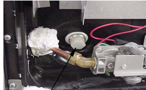
Water Heater Drain Plug (Remove with socket)
