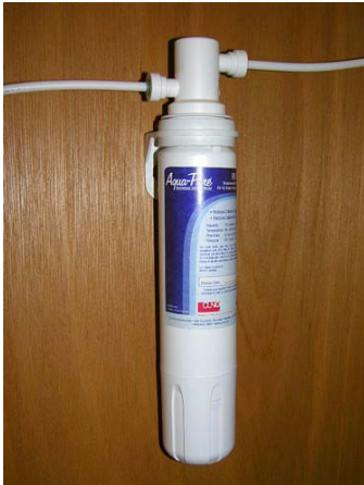
Water Filter Assembly (Located below Galley Sink)
