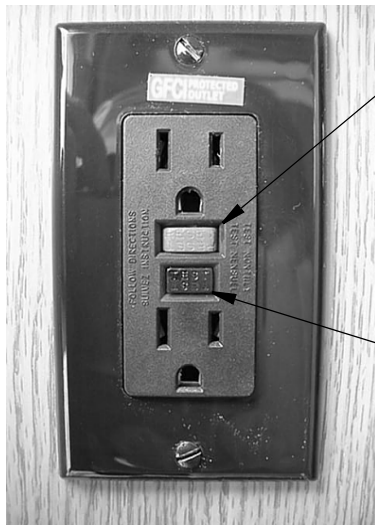
GFCI Outlet (Ground Fault Protector)
