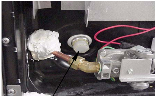
Water Heater Drain Plug (Remove with socket)
