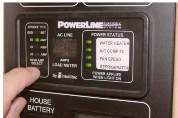
PowerLine EMS Display on Monitor Panel - typical
