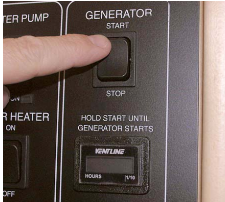
Generator Switch and Hourmeter on monitor panel
