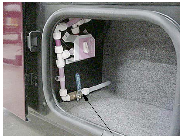
Water Line Drain Valve in RH Exterior Compartment (additional on Model 40KD only)
