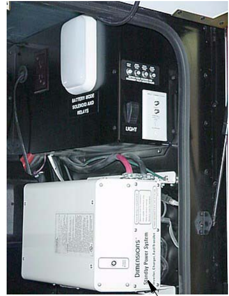
Inverter Charger Unit Location in utility compartment
