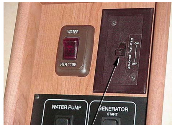
Diesel Engine Heater Switch (typical)
