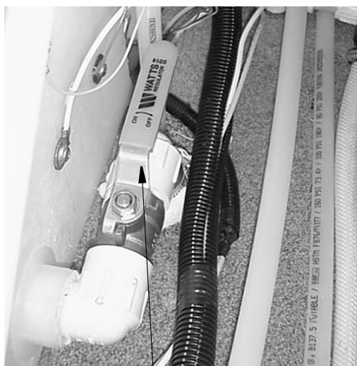
Water Tank Drain Valve (Typical)
