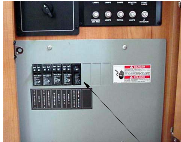
120-Volt House Circuit Breakers
