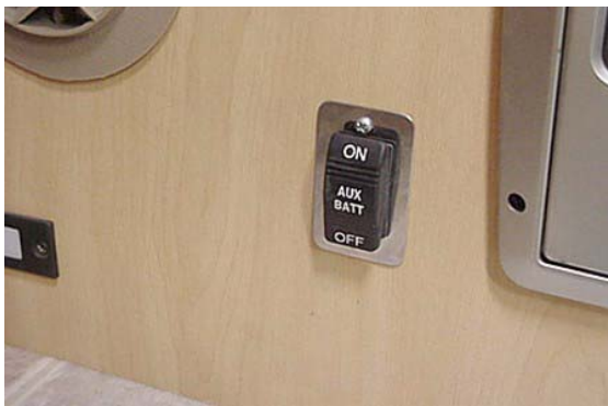
Aux. Batt. Switch - typical (Near entrance door)
