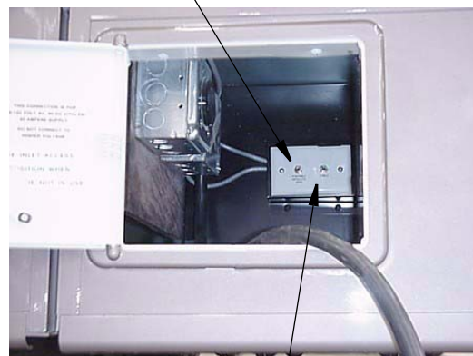
Portable Satellite Dish Hook-up in Shoreline Compartment
