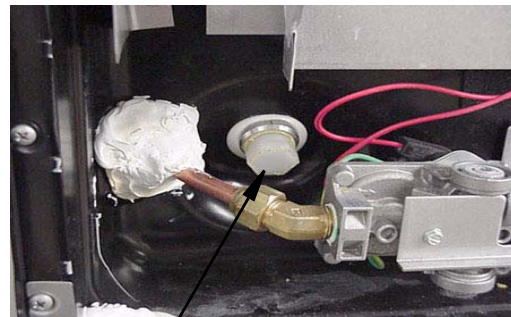
Water Heater Drain Plug Remove with socket
