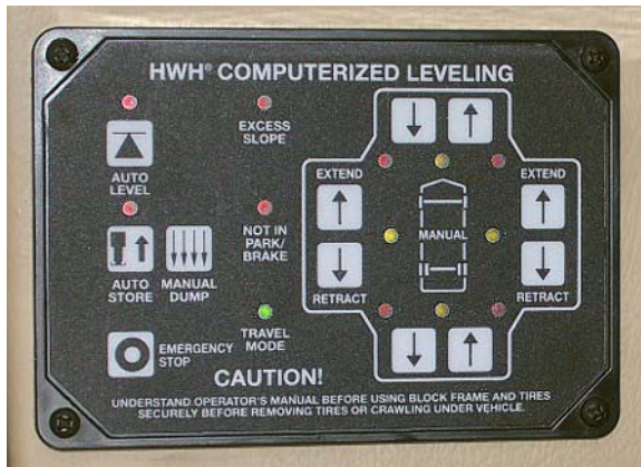
Leveling System Control Panel
