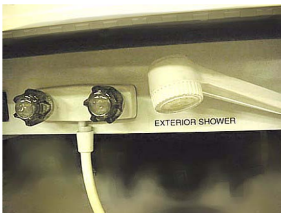
Exterior Shower/Wash Station (Typical)
