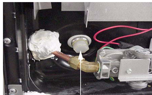
Water Heater Drain Plug (Remove with socket)
