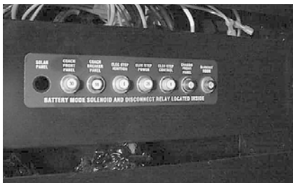
Chassis and House 12V Breakers (cover off)
