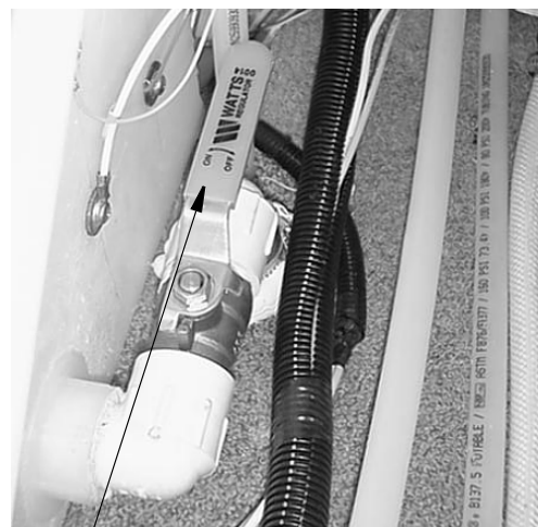
Water Tank Drain Valve
