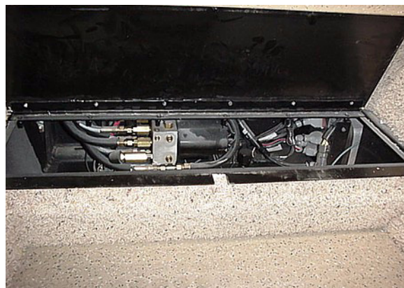
Hydraulic Pump beneath Entry Step
