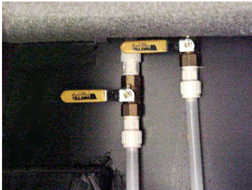
Water Line Drain Valves in Water Center
