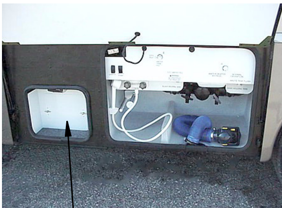
Water drain valves located behind access panel
