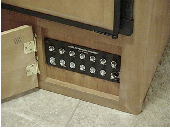
House 12-Volt Circuit Breaker Panel - typical*
