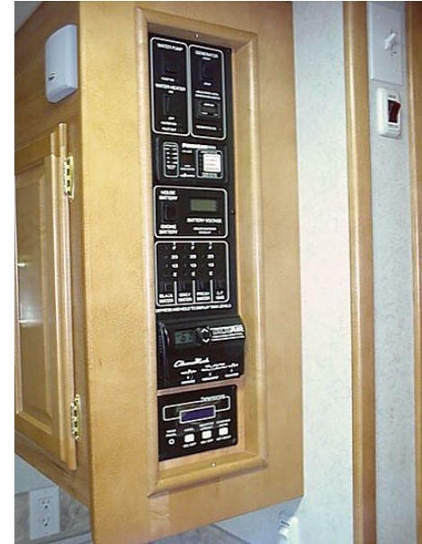
One Place Monitor Panel
