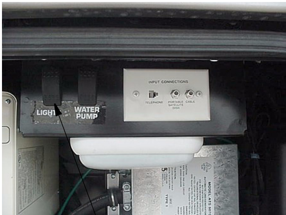
Utility Light Switch
