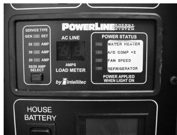
PowerLine EMS Display on OnePlace Monitor Panel
