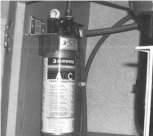
Water Filter Assembly below galley sink
