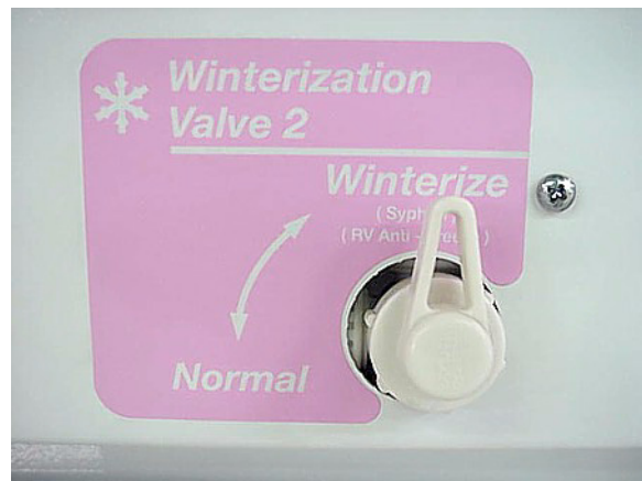
Winterization Valve in water service center
