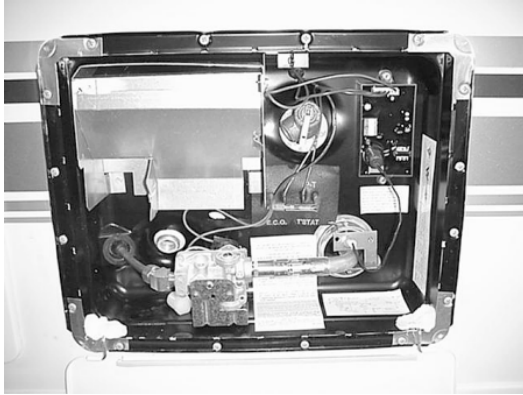
Water Heater Exterior Service Access
