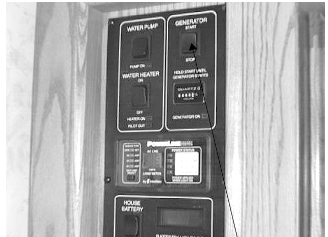
Generator Switch and Hourmeter
