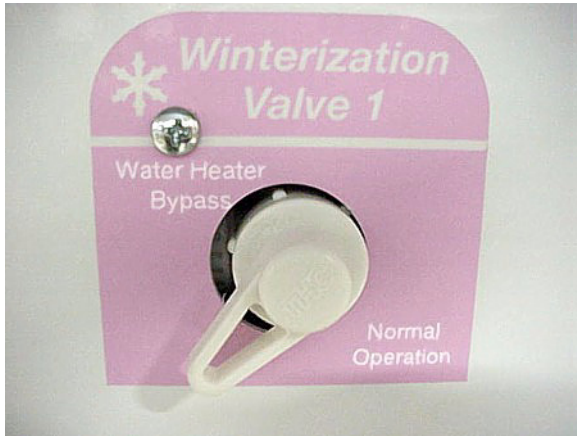
Water Heater By-Pass Valve
