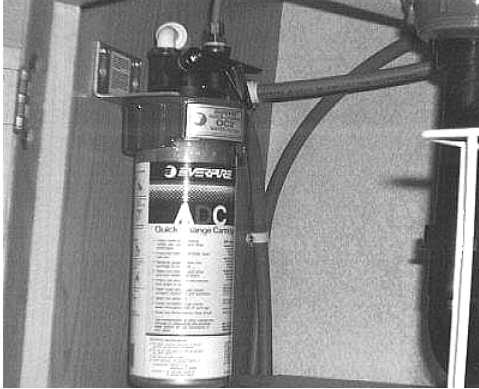
Water Filter Assembly below Galley Sink
