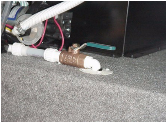
Water Line Drain Valve in RH Exterior Water Pump Compartment
