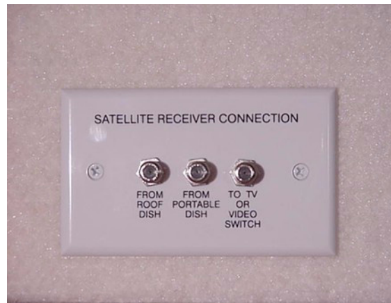
Interior Connection for Satellite Receiver (in front left video center cabinet)
