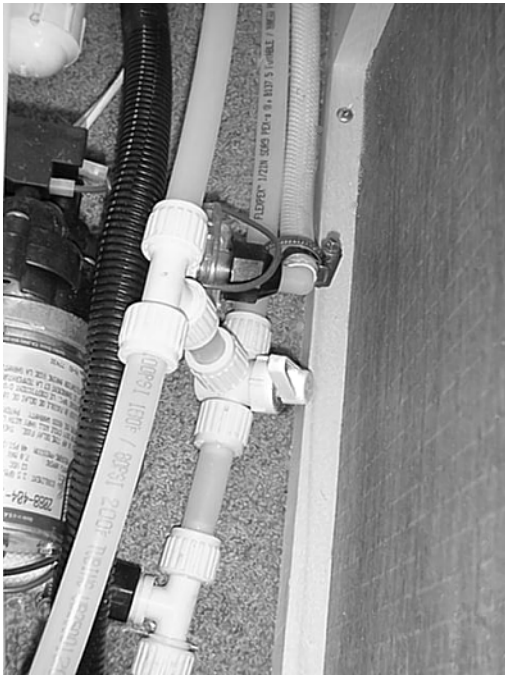
Water Heater By-Pass Valve (Typical) Beneath Bed
