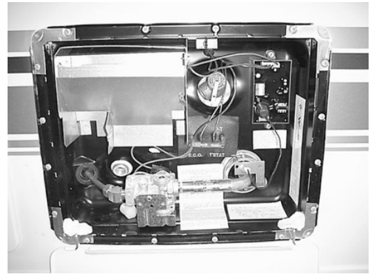
Water Heater Exterior Service Access
