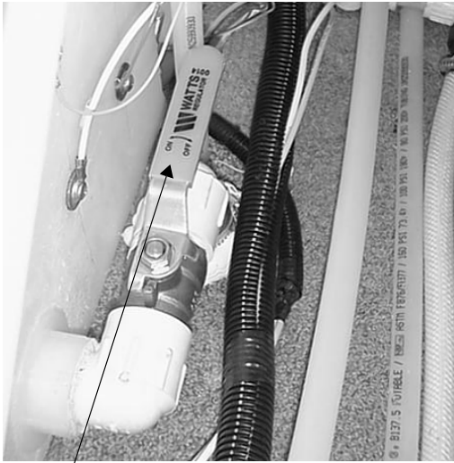
Water Tank Drain Valve (Typical)
