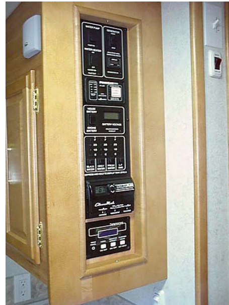
One Place Monitor Panel
