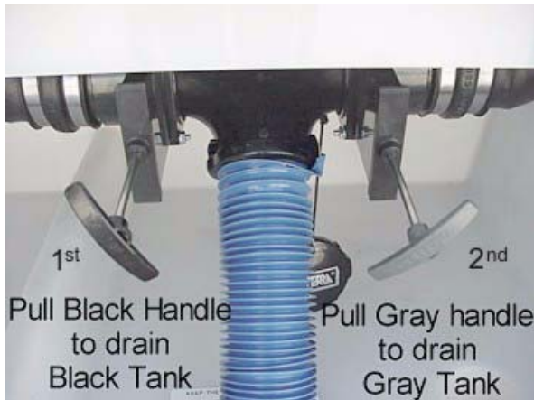
Holding Tank Valves (Typical)
