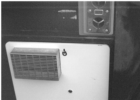
Water Heater Service Access Panel
