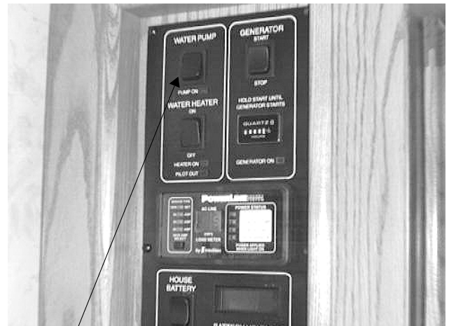
Water Pump Switch
