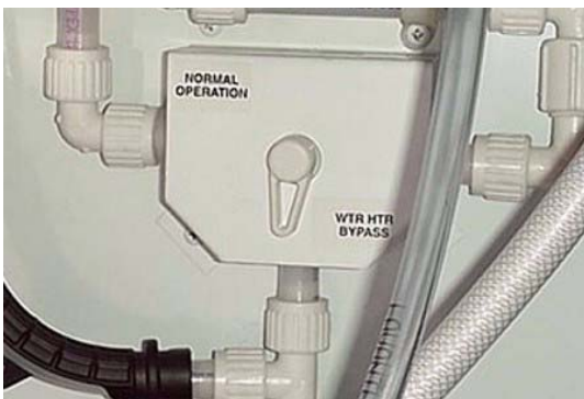
Water Heater By-Pass Valve (Typical)
