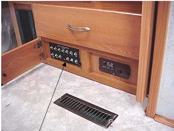
House 12-Volt Circuit Breaker Panel
