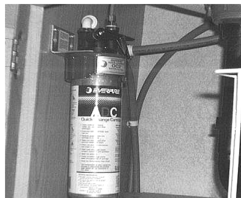
Water Filter Assembly - Below Galley Sink
