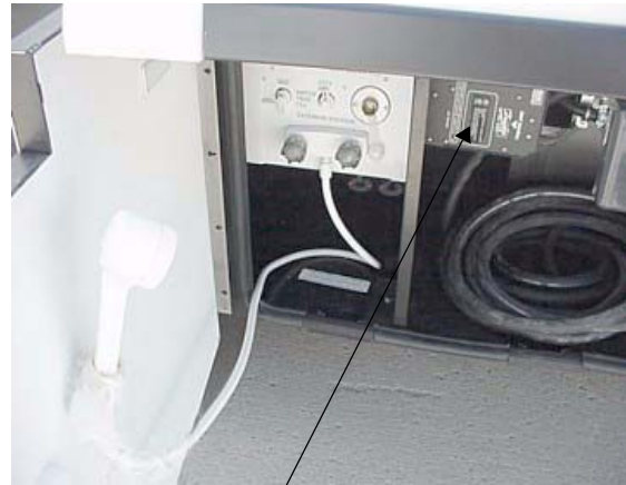
Inverter Charger Unit Location in shoreline compartment
