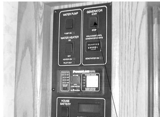
Generator Switch and Hourmeter
