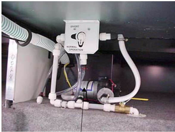
Water Pump (typical)
