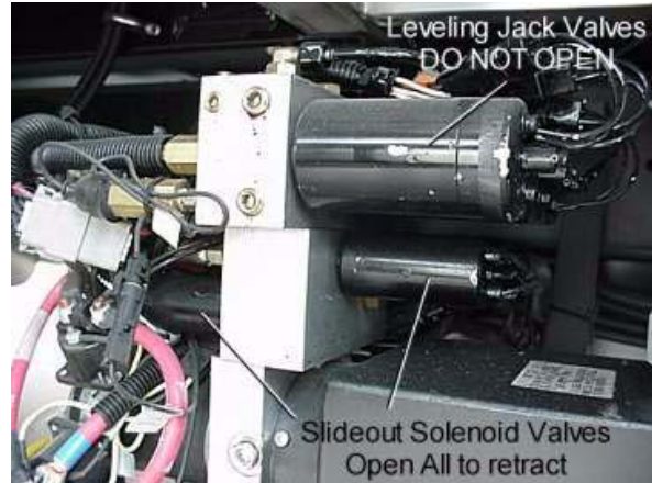
Leveling/Slideout System Hydraulic Pump (Note valve positions in relation to fluid reservoir)
