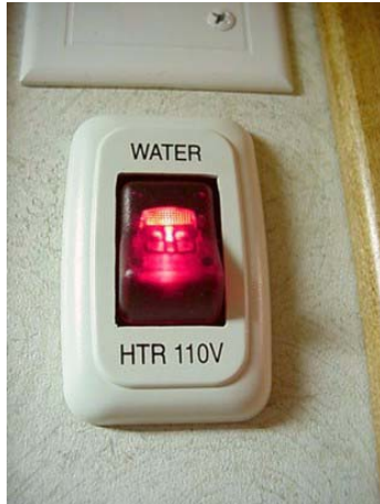
Electric Water Heater Switch (Typical)
