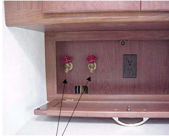
Water Supply Faucets Typical
