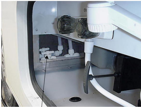
Hot and Cold Water Line Drains (in front of water service center)
