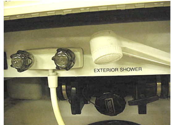
Exterior Shower/Wash Station
