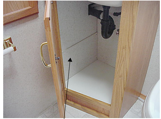
Water Heater Bypass Valve behind Access Panel beneath Bath Lavatory Vanity
