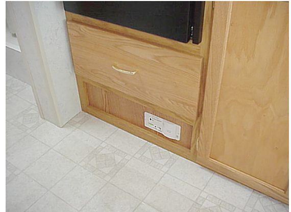
LP Gas Leak Detector
