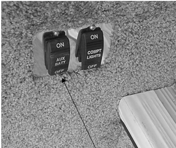
Aux. Batt. Switch (Near entrance door)
