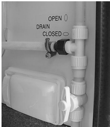
Water Line Drain in right front compartment
