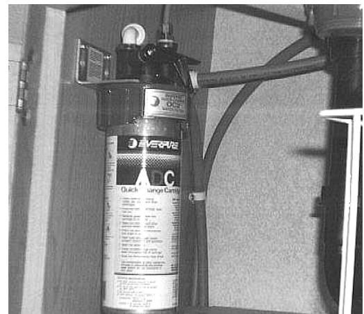
Water Filter Assembly - Below Galley Sink
