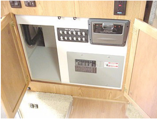
110-Volt Circuit Breaker Panel
