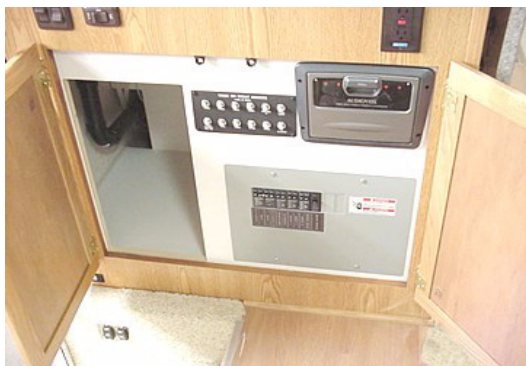
House 12V Circuit Breakers
