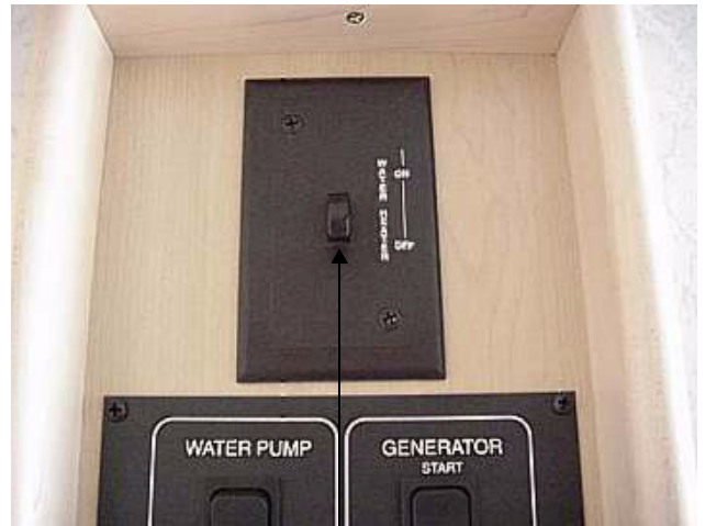
Electric Water Heater Switch above monitor panel.
