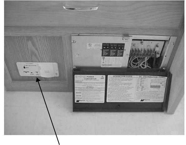
LP Gas Alarm
