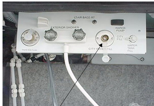
City Water Connection
