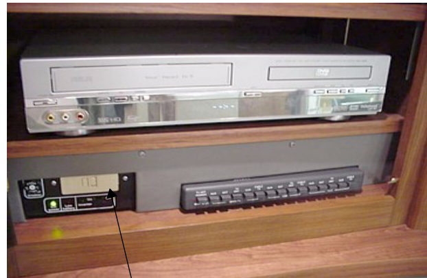
DC-AC Voltage Inverter in Video Center
