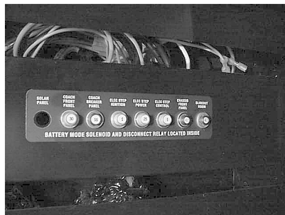
Chassis and House 12V Circuit Breakers in cargo compartment near entrance door
