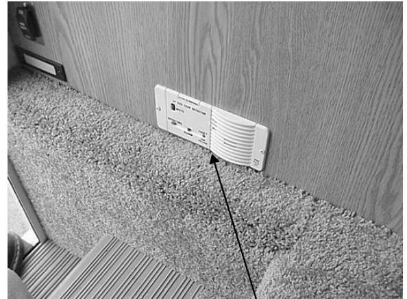
LP Gas Alarm
