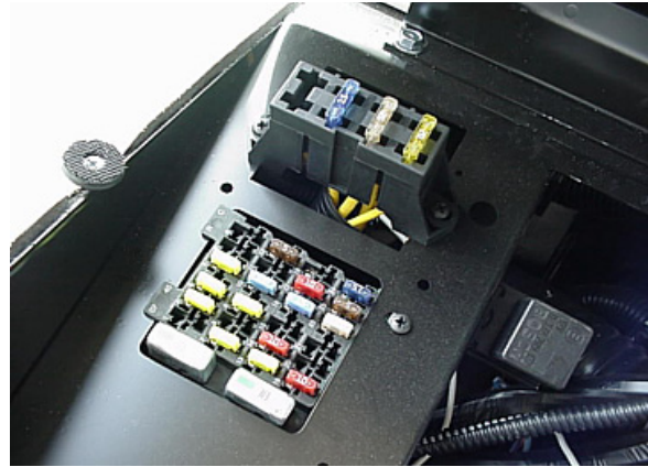
Automotive 12-Volt Fuse Block (Under lift-up dash pod)
