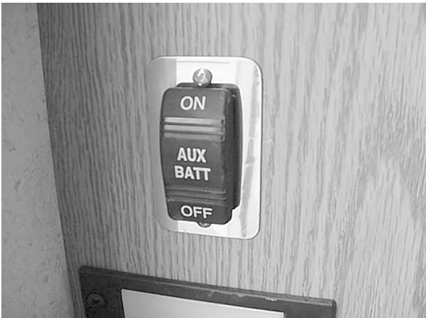
Aux. Batt. Switch (Near entrance door)
