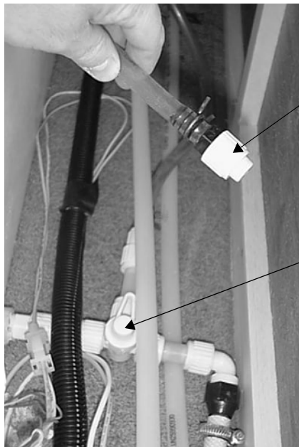
Winterization Valve beneath rear bed
