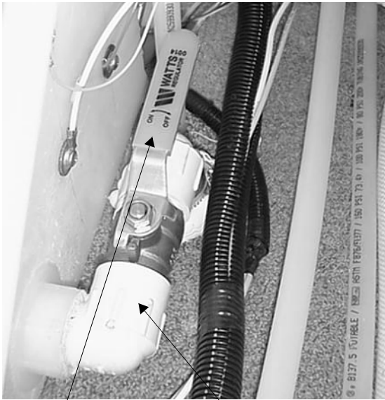
Water Tank Drain Valve Winterization Valve
