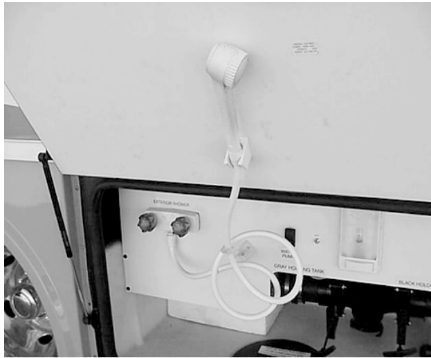
Exterior Shower/Wash Station (Typical)
