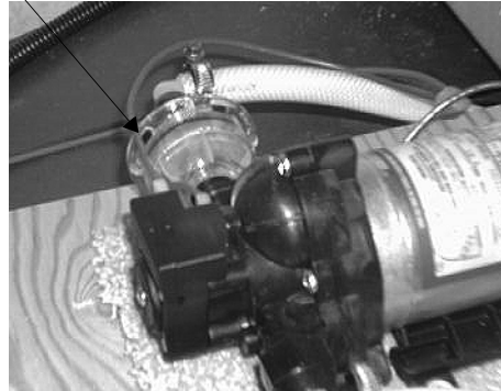
Water Pump and Filter
