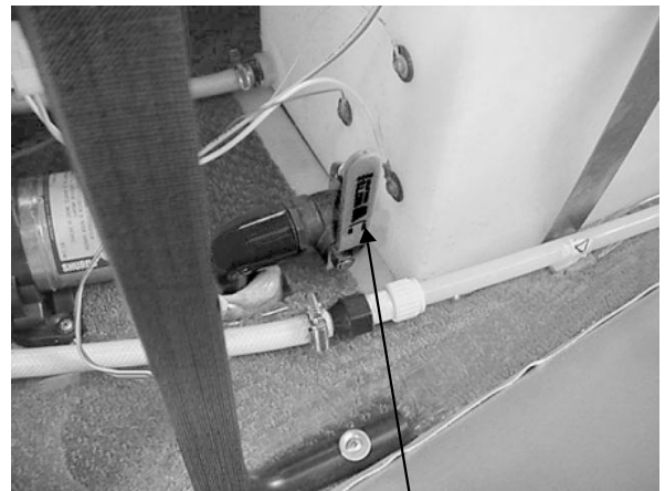
Water Tank Drain Valve
