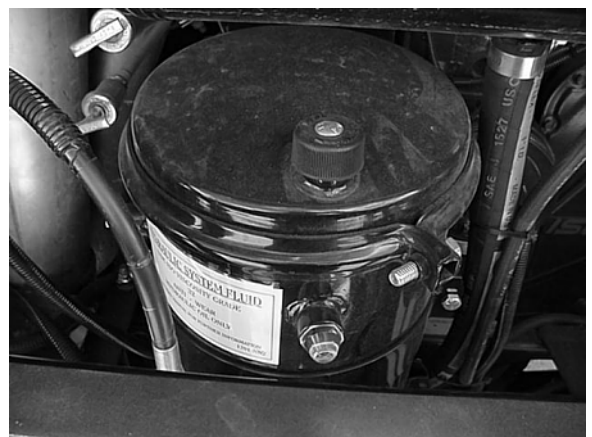
Hydraulic Fluid Tank
