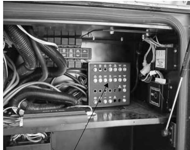
Automotive 12-Volt Breaker Panel
