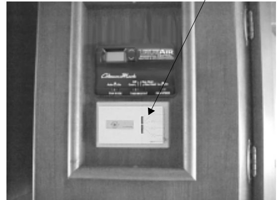
Power Ventilator Thermostat - Galley
