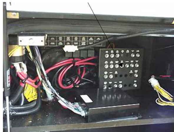
Automotive/Chassis Electrical Center (Left Front Compartment)
