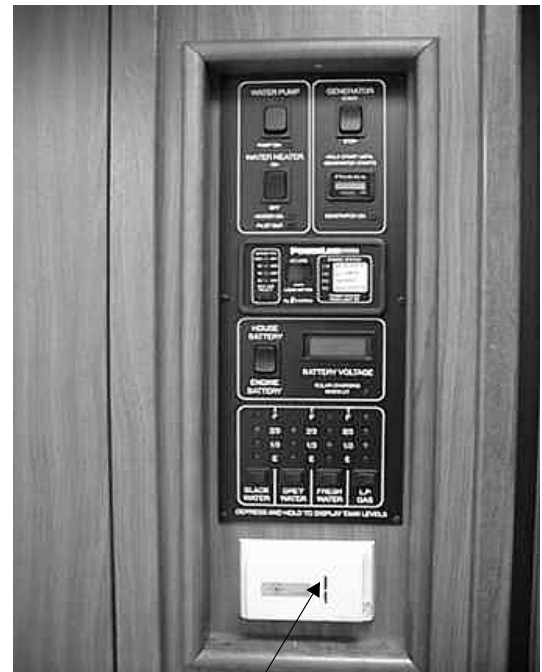
Power Vent Thermostat Bath Area
