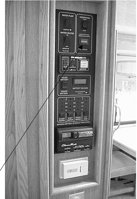
Generator Switch and Hourmeter
