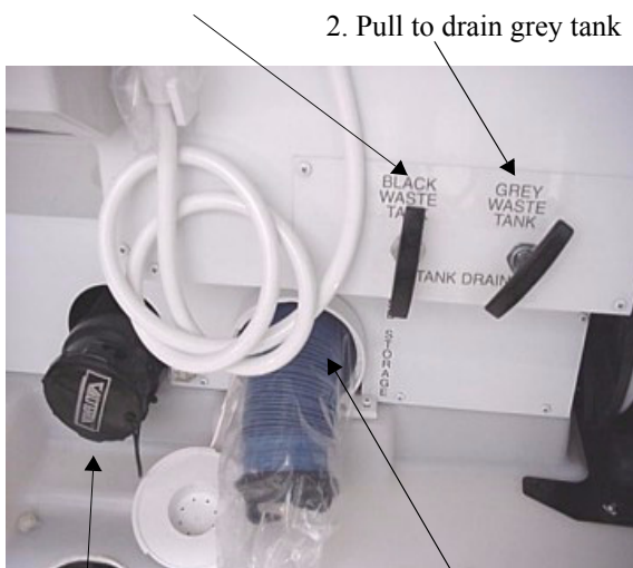
Waste Drain Outlet
