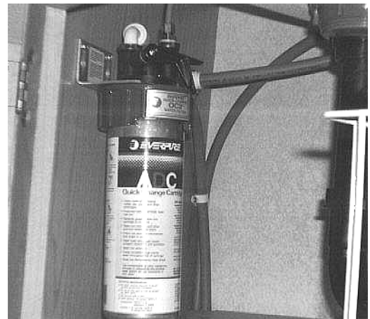
Water Filter Assembly - Below Galley Sink
