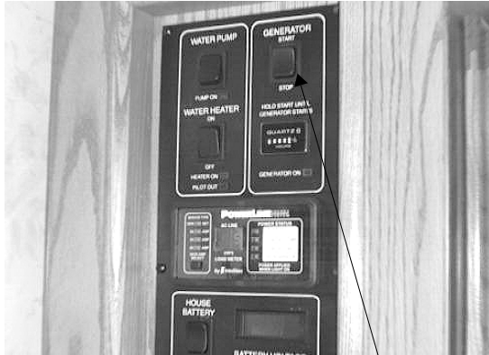
Generator Switch and Hourmeter
