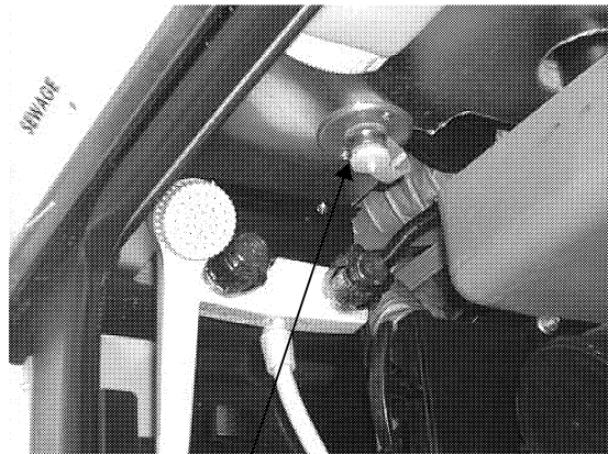
City Water Connection
