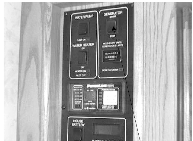
Generator Switch and Hourmeter
