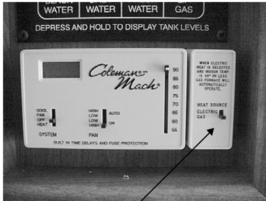
Heat Source Switch ELECTRIC = Heat Pump GAS = Furnace
