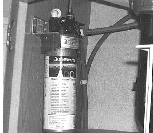
Water Filter Assembly - Below Galley Sink
