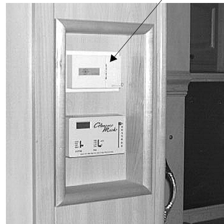
Power Ventilator Thermostat - Galley
