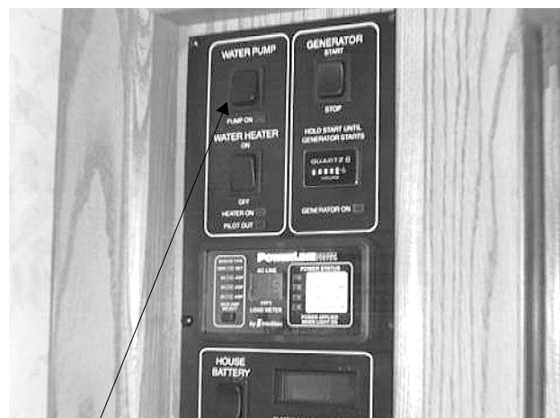
Water Pump Switch
