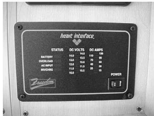
Inverter/Charger Remote Panel
