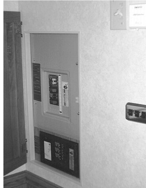
110-Volt Circuit Breakers behind door on bedroom forward wall
