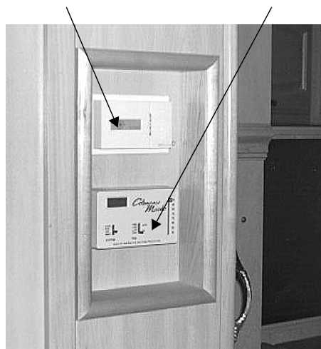
Power Ventilator Thermostat Heating/Cooling Thermostat
