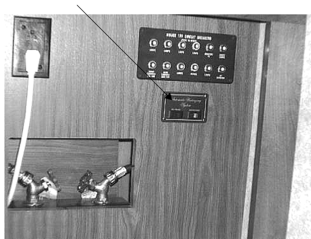
Winterization System Switches
