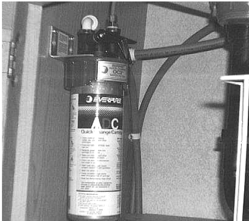
Water Filter Assembly - Below Galley Sink
