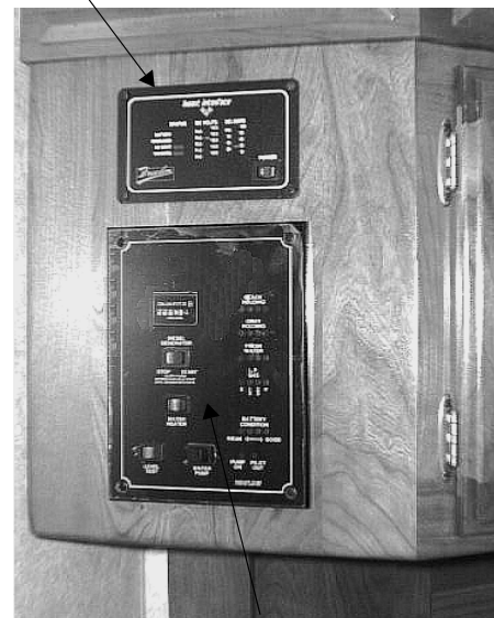
Main System Monitor Panel
