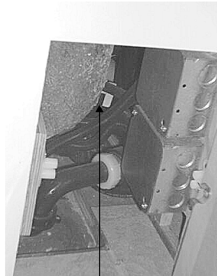
Shower Line Drain Valve (shown exposed with access panel removed)
