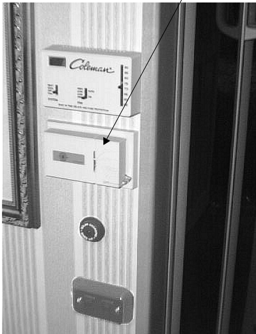
Power Ventilator Thermostat - Galley
