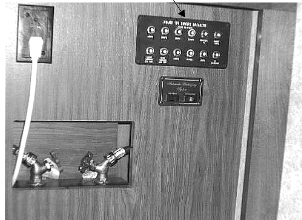
House 12-Volt Circuit Breaker Panel
