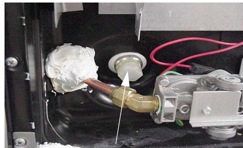
Water Heater Drain Plug (Remove with socket)
