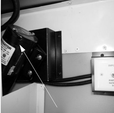
Waste Pump (Located behind water service center - accessible through utility compartment) -Typical View
