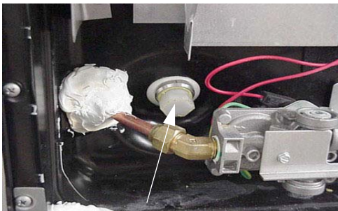
Water Heater Drain Plug (Remove with socket)
