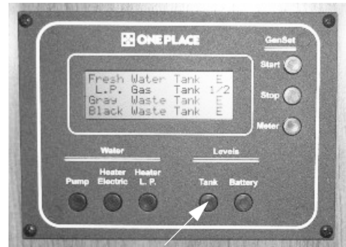
Tank Levels Switch
