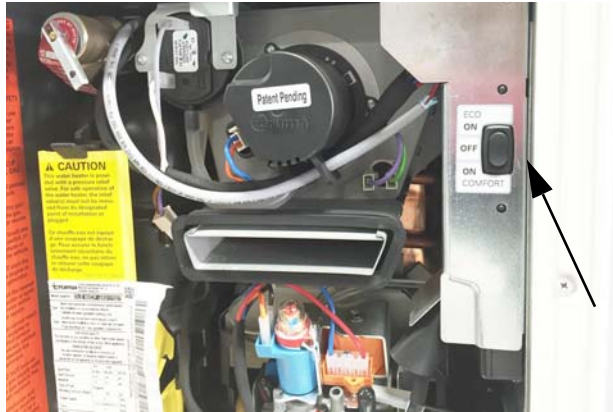
Water Heater Power Switch (Located behind water heater access panel on exterior of coach)
