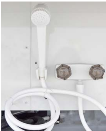
Exterior Shower/Wash Station -Typical View
