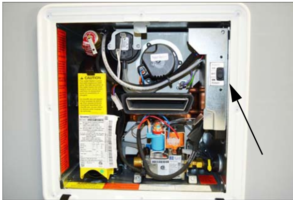
Water Heater Power Switch (Located behind water heater access panel on exterior of coach)
