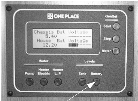
Battery Levels Switch
