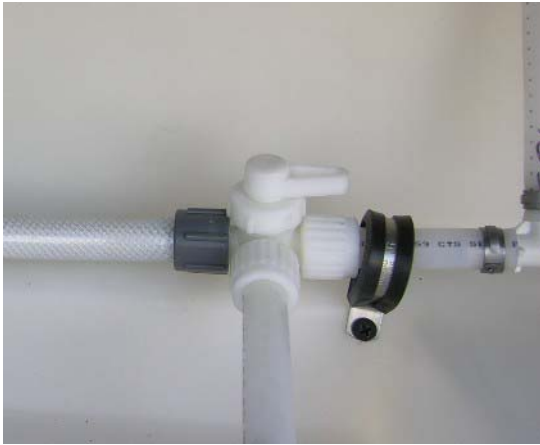
Waterline Drain Valve -Typical installation shown
