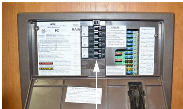
120-Volt Circuit Breakers -Typical View
