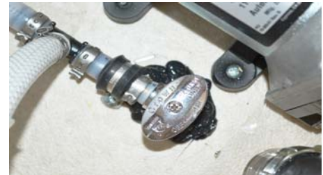
OFF ON Water Tank Drain Valve (Typical)
