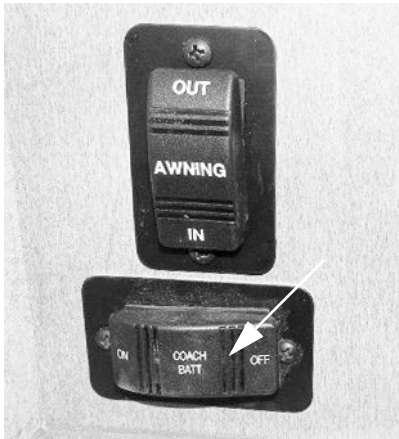
House/Coach Battery Disconnect Switch (Located near entrance door)
