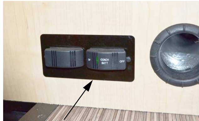
House/Coach Battery Disconnect Switch (Located near sliding door)
