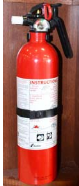
Fire Extinguisher (Located near sliding entrance door)
