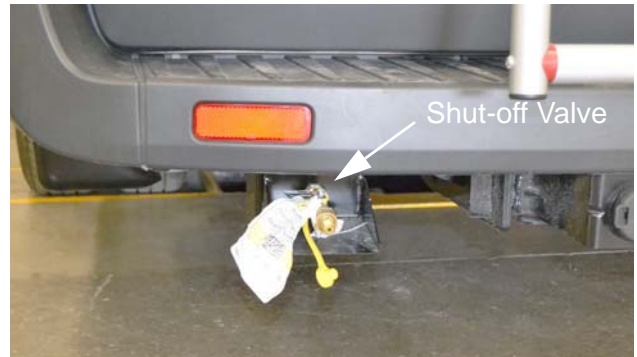
LP Accessory Connection (Located at rear of coach) -Typical View
