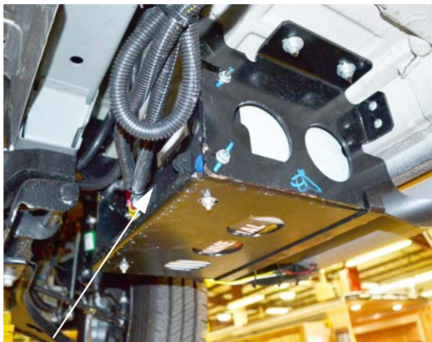
House Battery Access (Located below driver and passenger side cab door running boards)
