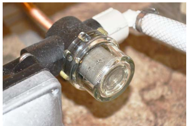
Shower Filter Screen (Located beneath wardrobe cabinet - remove drawers to access -Typical View
