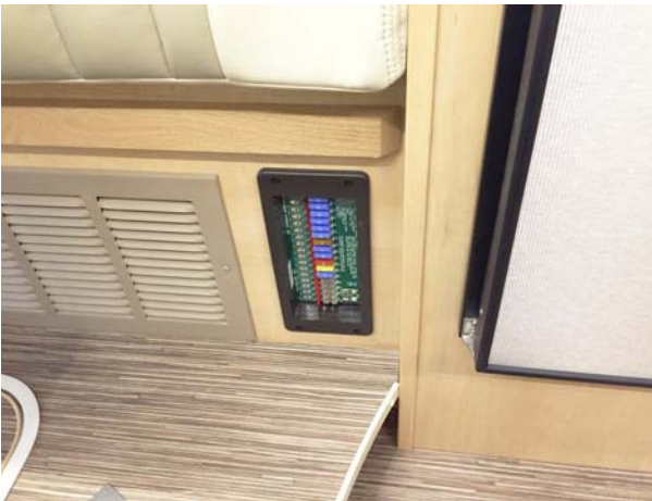
House 12-Volt Fuses (Located on driver side dinette cabinet) -Typical View
