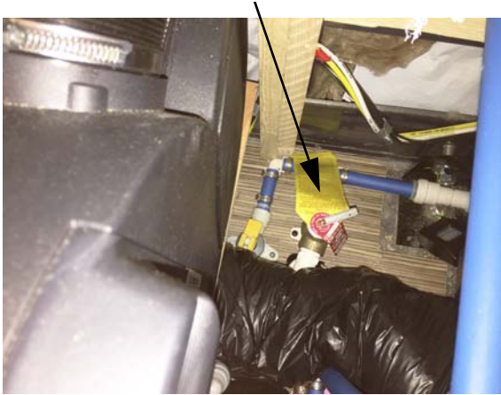
Pressure Temperature Relief Valve (Located beneath driver side dinette seat)
