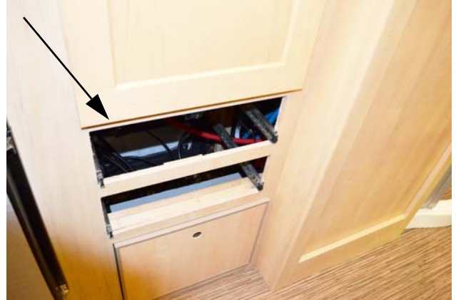
Shower Pump (Located beneath wardrobe cabinet - remove drawers to access -Typical View
