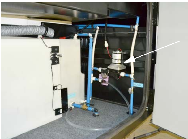
Water Pump (Located in a passenger side compartment) *38W Shown
