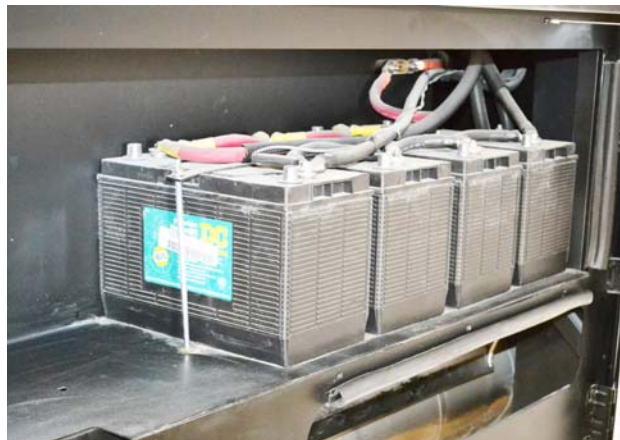
House/Coach Batteries -Typical View
