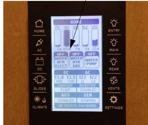
Water Heater Switch “HOME” Screen (Located on Multiplex Monitor Panel)
