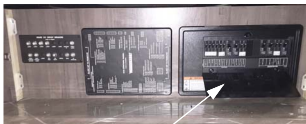
House Circuit Breakers -Typical Installation
