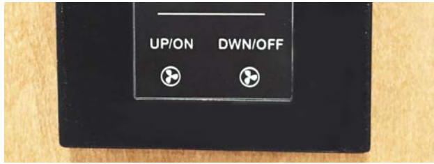
Power Roof Ventilator Switches
