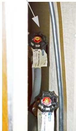
Water Supply Faucets (Located behind access panel within wardrobe) *Model 34T
