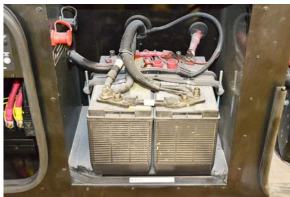
Chassis Batteries -Typical View
