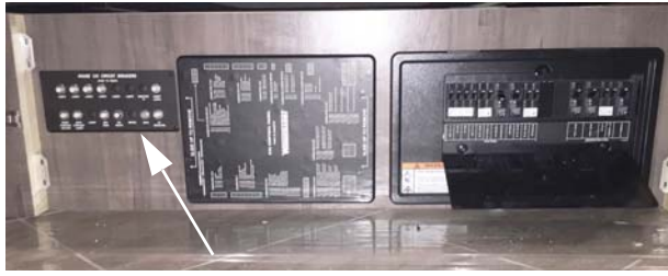
House Circuit Breakers -Typical View
