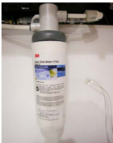
Cold Water Filter Assembly (Located below galley sink)
