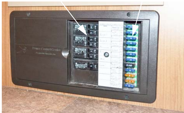
Power Center (Converter) -Typical View
