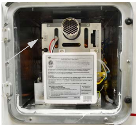
Water Heater Power Switch (Push to turn ON)
