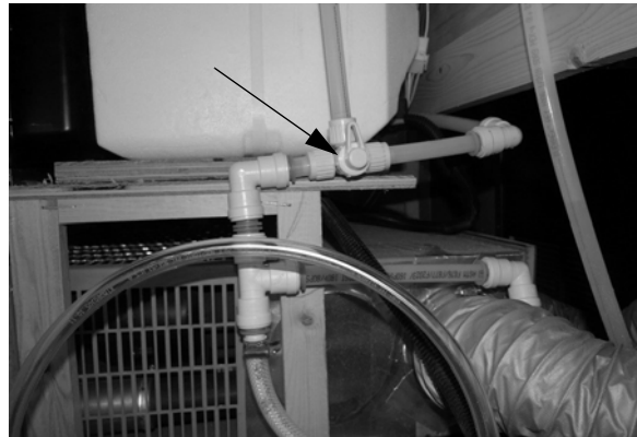
Water Heater Bypass Valve
