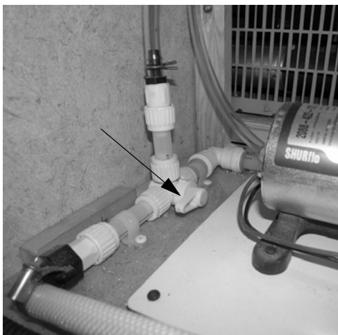
Winterization Valve -Typical View
