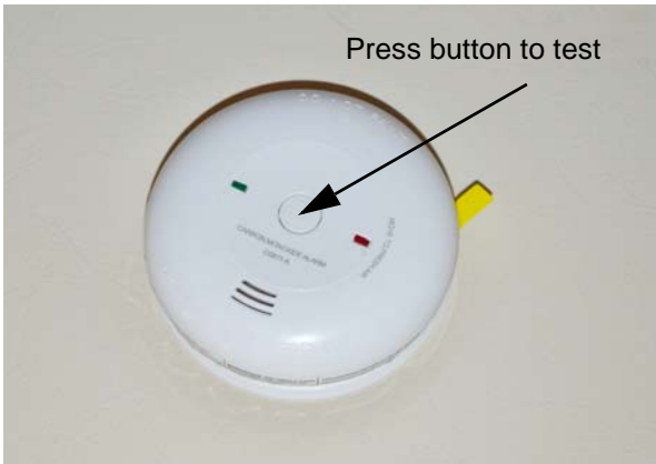
Carbon Monoxide Alarm
