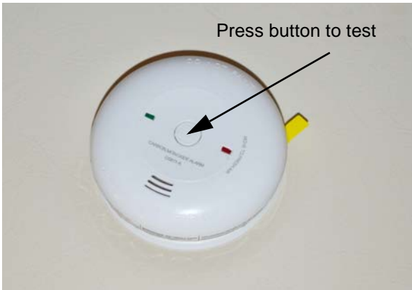
Carbon Monoxide Alarm
