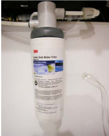
Galley Filtered Cold Water Faucet/ Ice Maker Filter Assembly (Located below galley sink) -Typical View
