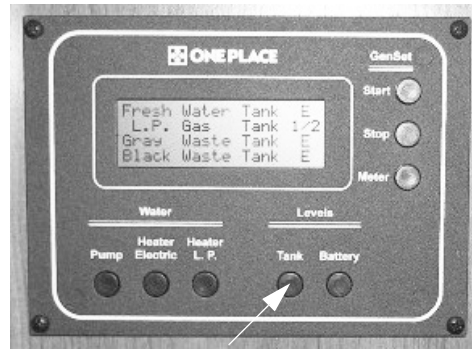
Tank Levels Switch
