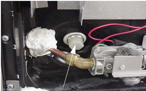
Water Heater Drain Plug (Remove with socket)
