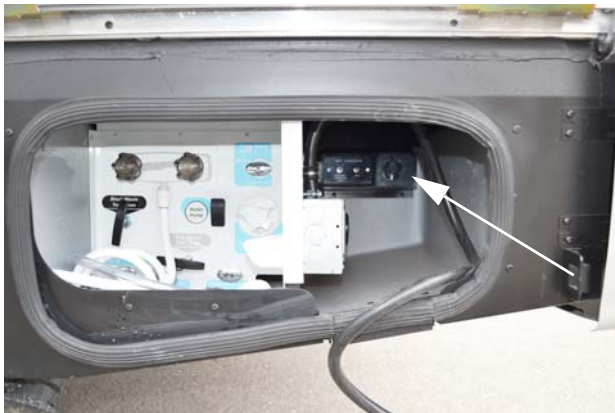
Single Solar Port (Located inside rear driver side exterior compartment)
