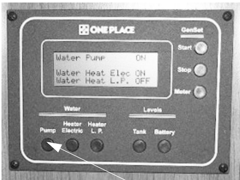
Water Pump Switch
