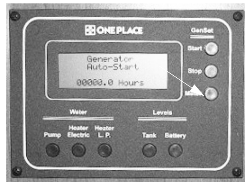
Generator Hourmeter Button -Typical View
