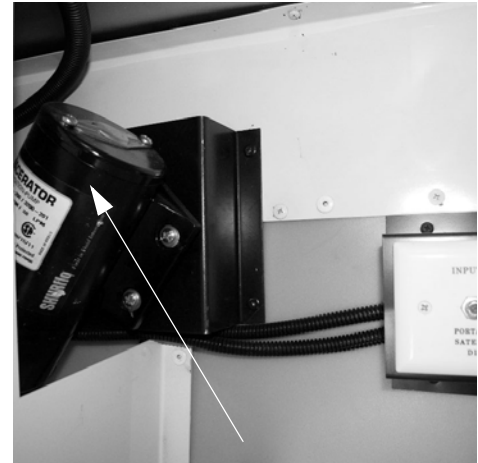
Waste Pump (Located behind water service center - accessible through utility compartment) -Typical View
