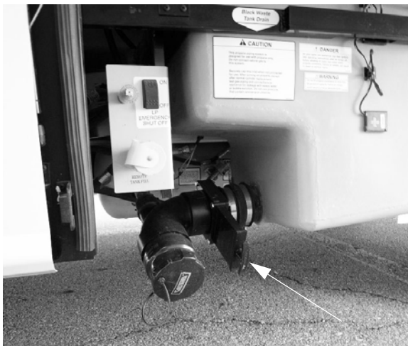
Black Waste Tank Drain Valve (Located in driver side compartment) -Typical View
