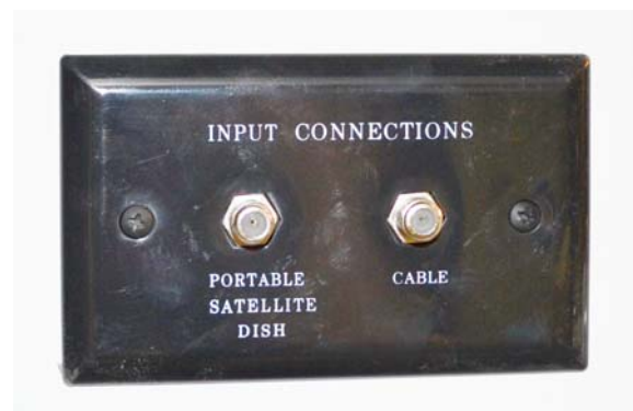
Cable TV and Portable Satellite Connections (Located in the utility or shoreline compartment depending on model.)
