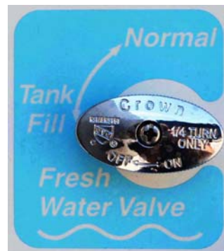
Fresh Water Valve (Located in water service center)
