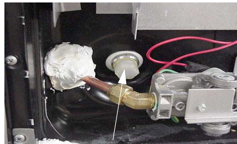
Water Heater Drain Plug (Remove with socket)
