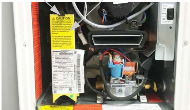
Easy Drain Lever (Located behind water heater access panel on exterior of coach)
