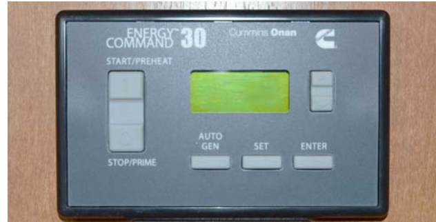
AGS Control Pad (Located near monitor panel)
