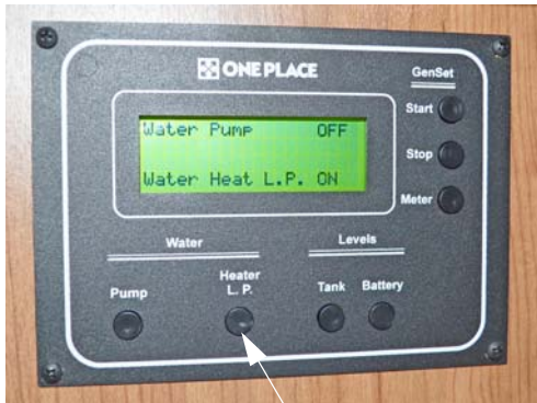
LP Gas Water Heater Switch
