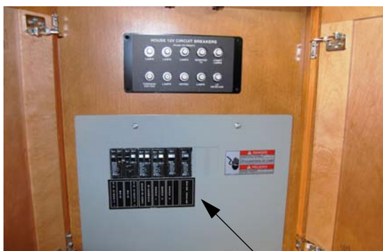
120-Volt House Circuit Breakers -Typical View
