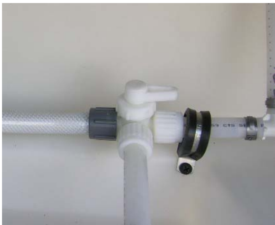
Waterline Drain Valve -Typical installation shown
