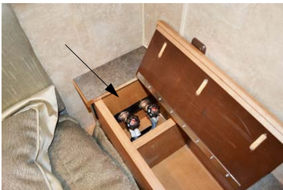
Water Supply Faucets (Located inside front nightstand)
