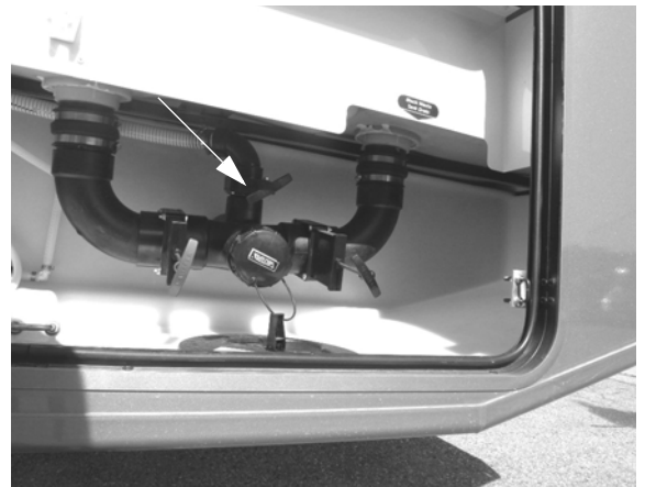
Black Waste Tank Drain Valve #2 (Front) (Located in water service center) -Typical View
