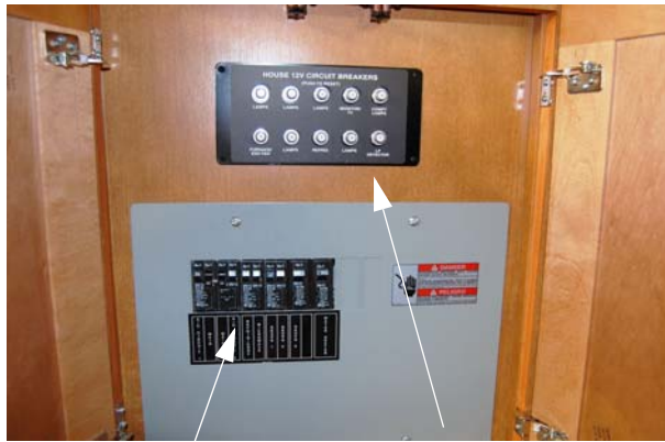
120-Volt House Circuit Breakers
