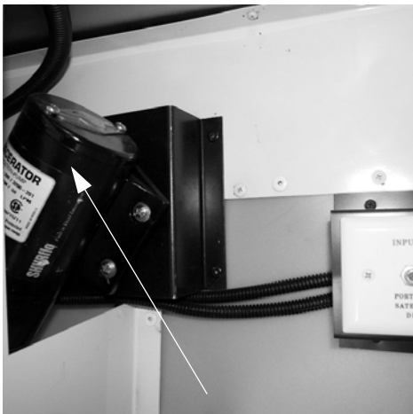
Waste Pump (Located behind water service center - accessible through utility compartment) -Typical View
