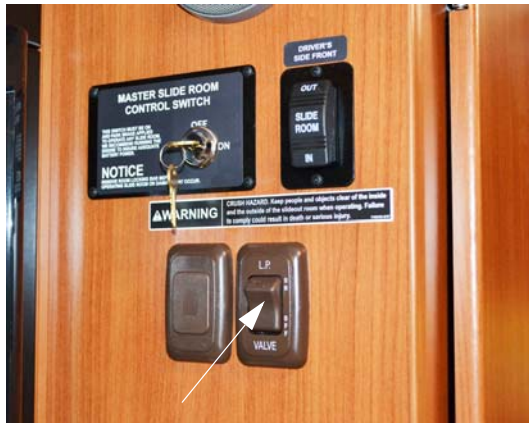
Main Tank Valve Switch (Located near monitor panel area) -Typical View
