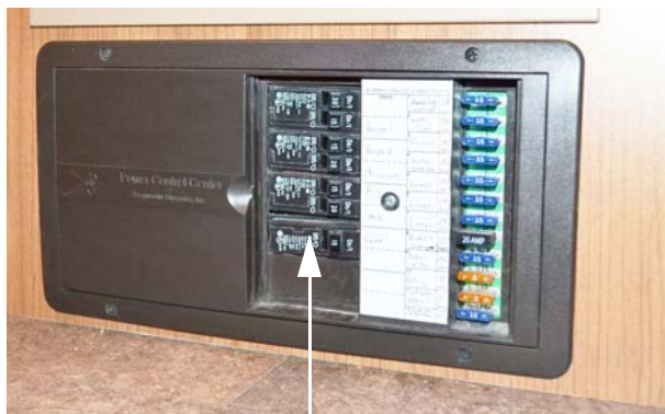
120-Volt Circuit Breakers -Typical View
