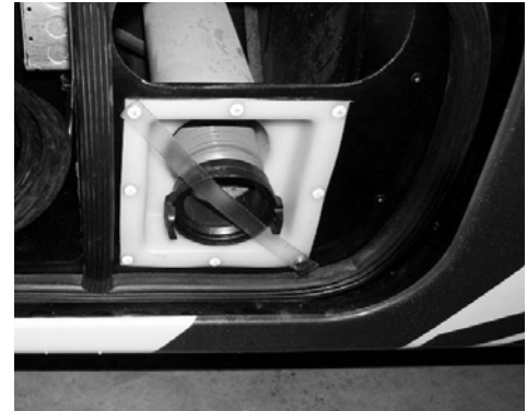
Sewage Drain Hose (Located in front driver side compartment) -Typical View
