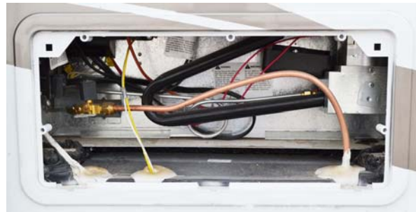
Refrigerator Access Compartment -Typical View
