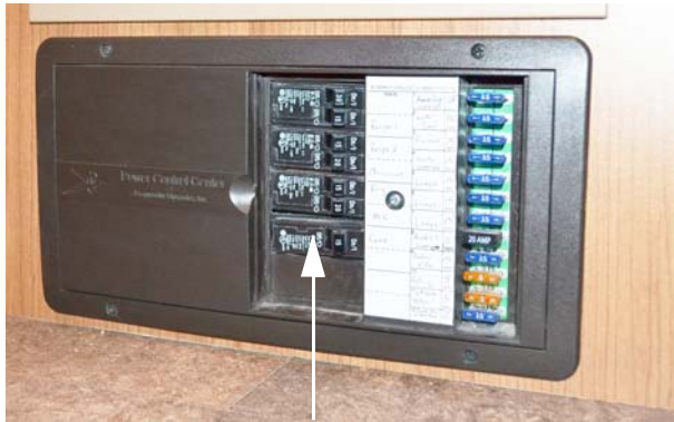
120-Volt Circuit Breakers -Typical View
