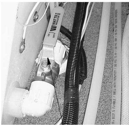
Water Tank Drain Valve (Typical)
