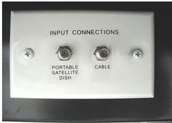
Cable TV and Portable Satellite Connections (Located in the utility compartment)
