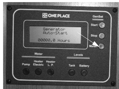
Generator Hourmeter Button -Typical View
