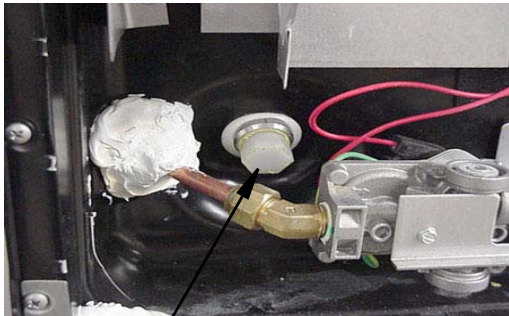
Water Heater Drain Plug (Remove with socket)
