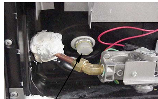
Water Heater Drain Plug (Remove with socket)
