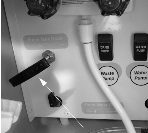
Water Tank Drain Valve -Typical View
