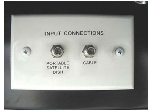
Satellite Dish and Cable TV Connections (Located in utility compartment or water service center) -Typical View
