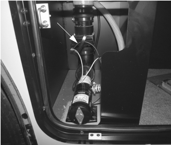
Black Waste Tank Drain Valve #1 (Front) (Located in passenger side compartment ahead of rear axle) -Typical View
