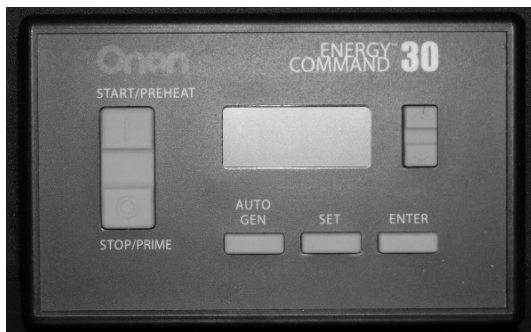
AGS Control Pad (Located near monitor panel)
