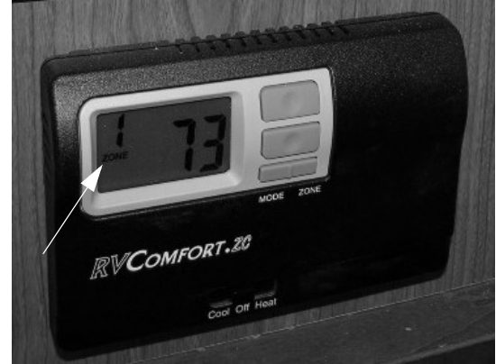
Zone 1 Operation (Living Area/Galley)
