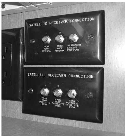
Interior Connection for Satellite Dish (Located near entertainment center cabinet) -Typical View
