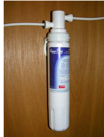
Filtered Water Faucet/Ice Maker Filter Assembly (Located below galley sink)
