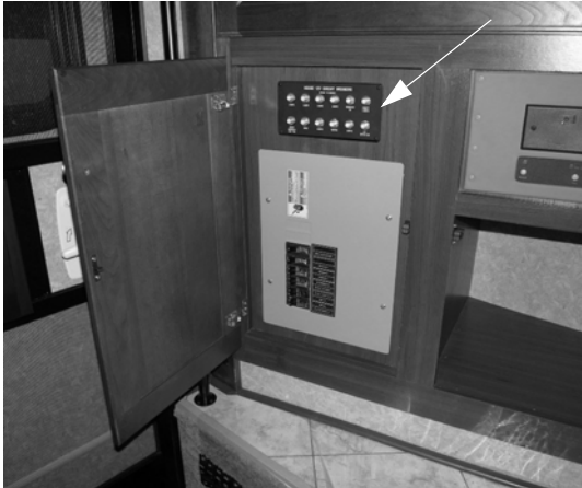
House 12V Circuit Breaker Panel -Typical View
