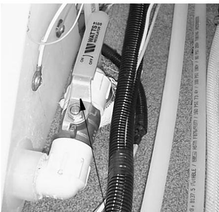
Water Tank Drain Valve (Typical)
