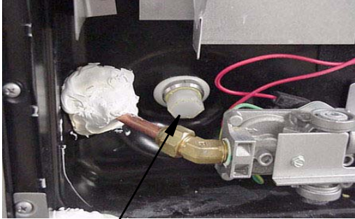
Water Heater Drain Plug Remove with socket
