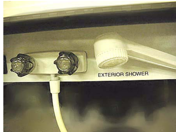
Exterior Shower/Wash Station -Typical View
