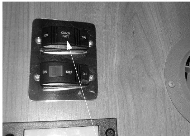
House/Coach Batt Disconnect Switch (Located near entrance door or end of galley, depending on model) -Typical View
