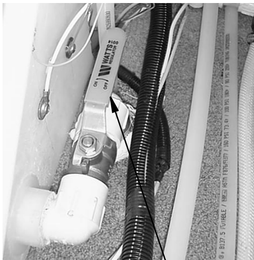
Water Tank Drain Valve (Typical)
