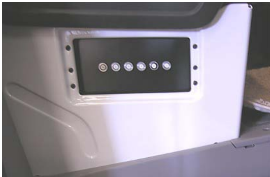
Chassis and House 12V Breakers on side of passenger seat base toward door (shown w/cover off)
