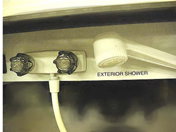
Exterior Shower/Wash Station -Typical View
