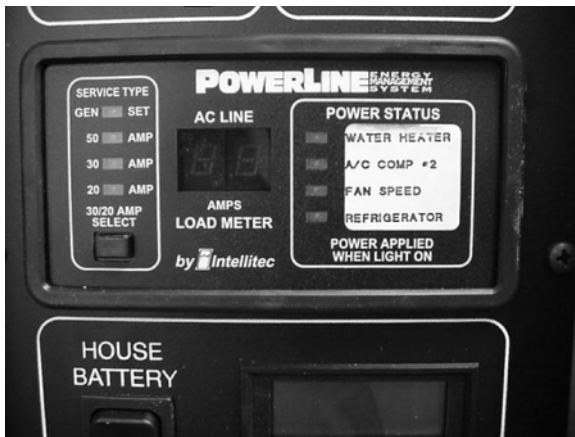
EMS Display on Monitor Panel (Typical View)
