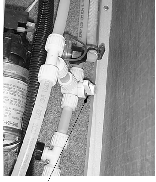
Water Heater Bypass Valve (Typical)
