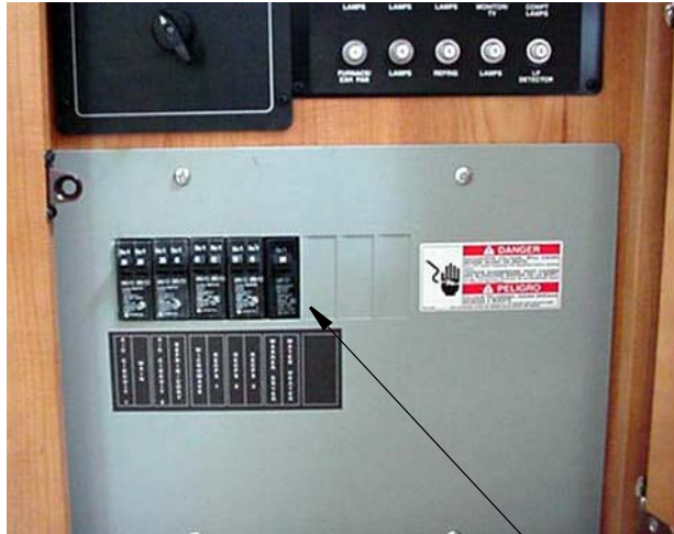
120-Volt House Circuit Breakers
