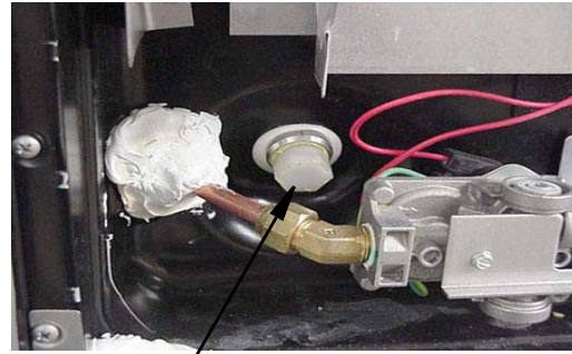
Water Heater Drain Plug Remove with socket
