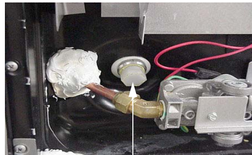
Water Heater Drain Plug (Remove with socket)
