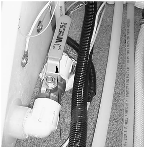
Water Tank Drain Valve (Typical)
