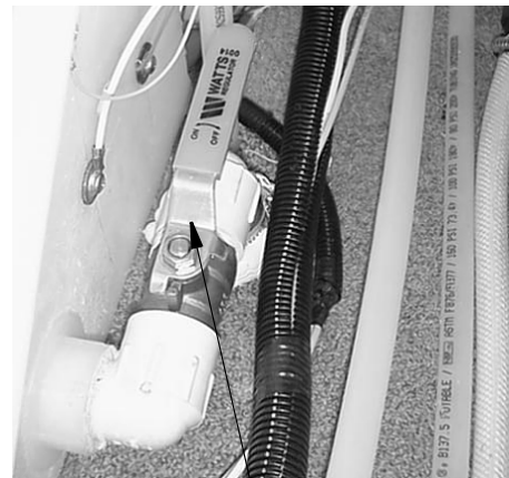
Water Tank Drain Valve (Typical)
