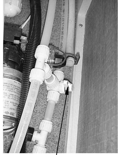
Waterline Drain Valve (Typical)
