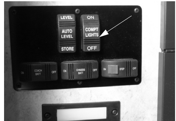
Compartment Lights Switch - Typical View (Located near entrance door)
