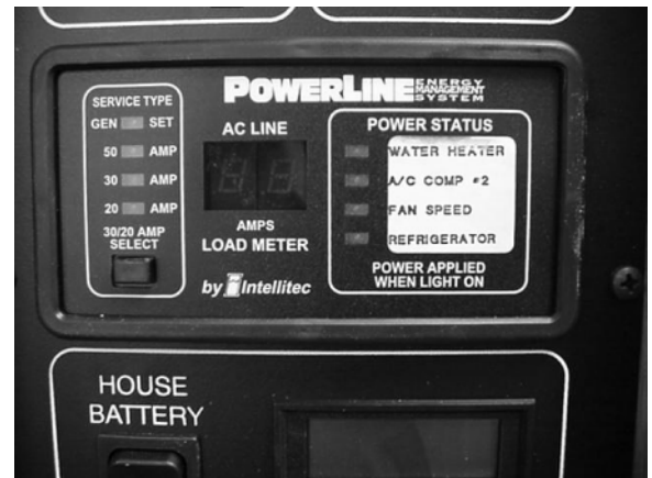
EMS Display on Monitor Panel -Typical View
