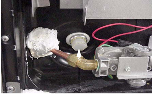
Water Heater Drain Plug (Remove with socket)
