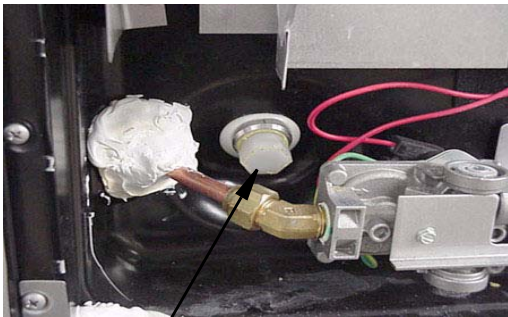
Water Heater Drain Plug (Remove with socket)
