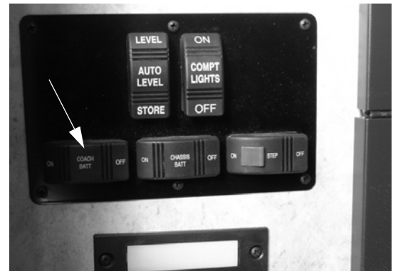
House/Coach Battery Disconnect Switch (Located near entrance door)
