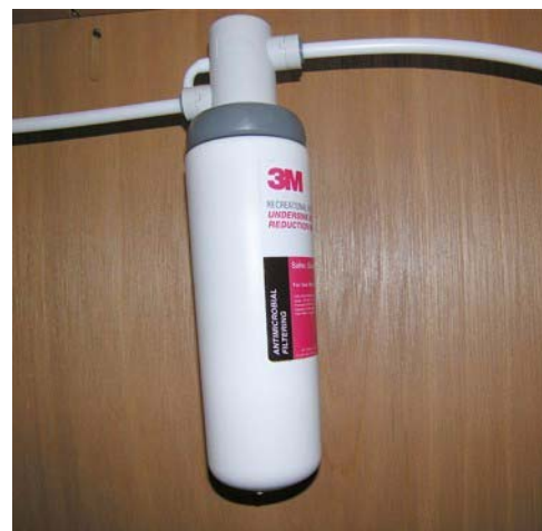
Cold Water Filter Assembly below Galley Sink (Hot water line is not filtered.)
