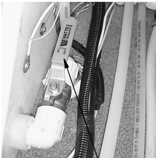
Water Tank Drain Valve (Typical)
