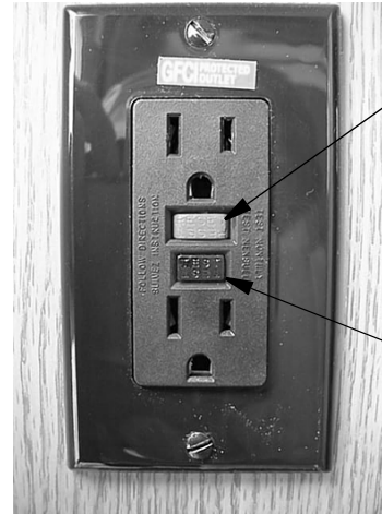
GFCI Outlet (Ground Fault Protector)
