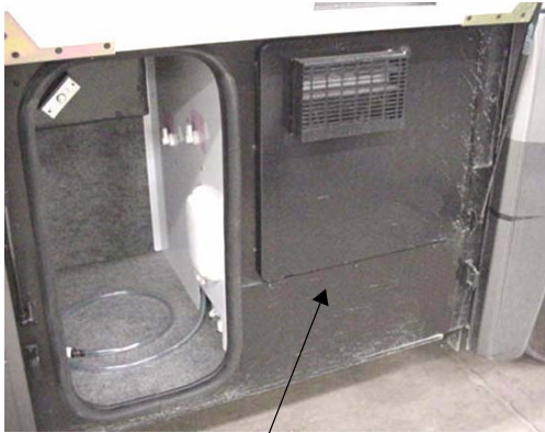
Water Pump Access Panel (typical)
