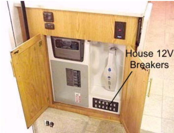
House 12-Volt Circuit Breaker Panel
