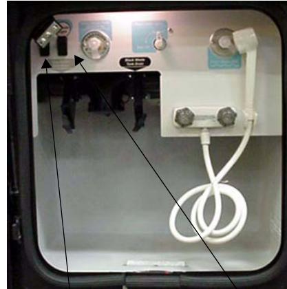
Utility Light Switch
