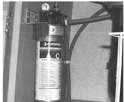
Water Filter Assembly - Below Galley Sink
