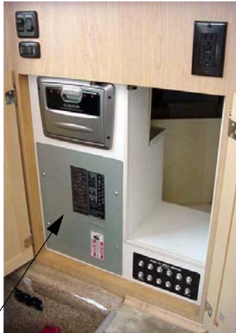
110-Volt House Circuit Breakers
