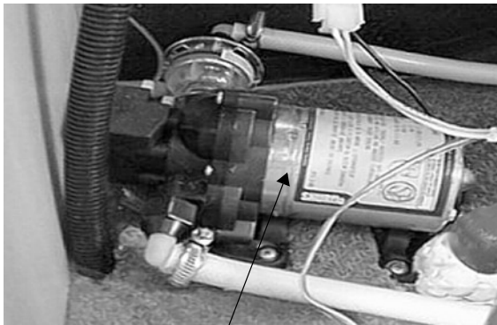
Water Pump (typical)
