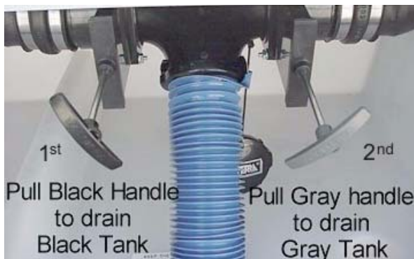
Holding Tank Valves (Typical)
