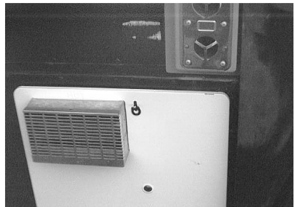
Water Heater Service Access Panel
