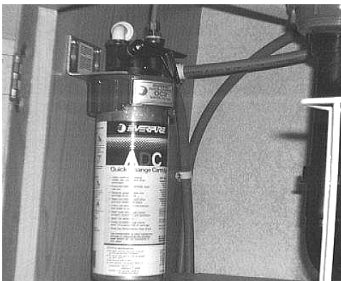
Water Filter Assembly - Below Galley Sink
