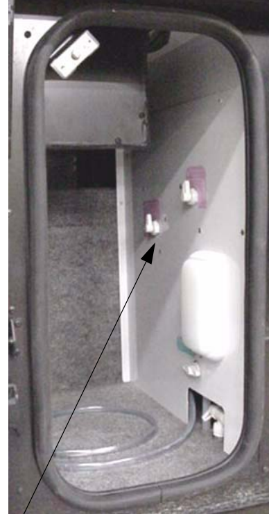
Water Heater Bypass Valve (Typical)
