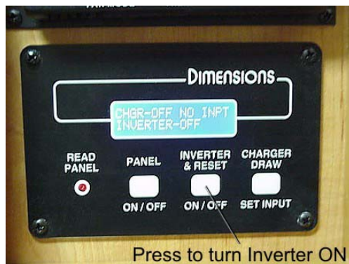
Inverter/Charger Control Panel
