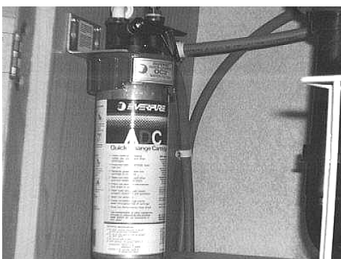
Water Filter Assembly below Galley Sink
