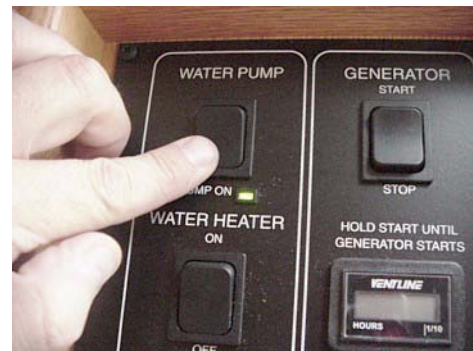
Water Pump Switch on OnePlace Panel
