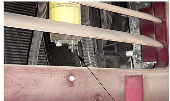
Fuel/Water Drain Valve
