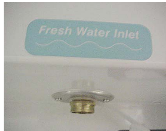
Fresh (City) Water Inlet
