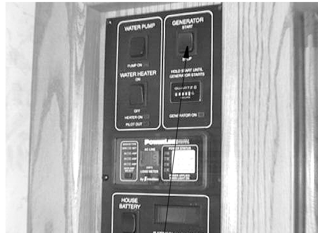
Generator Switch and Hourmeter
