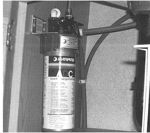
Water Filter Assembly below galley sink
