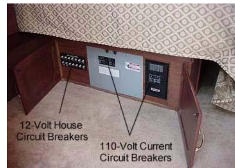
House 12V Breakers
