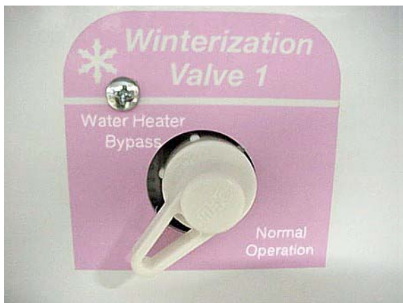
Water Heater By-Pass Valve
