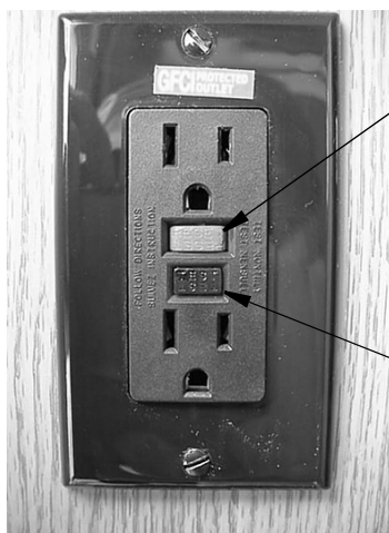
GFCI Outlet (Ground Fault Protector)
